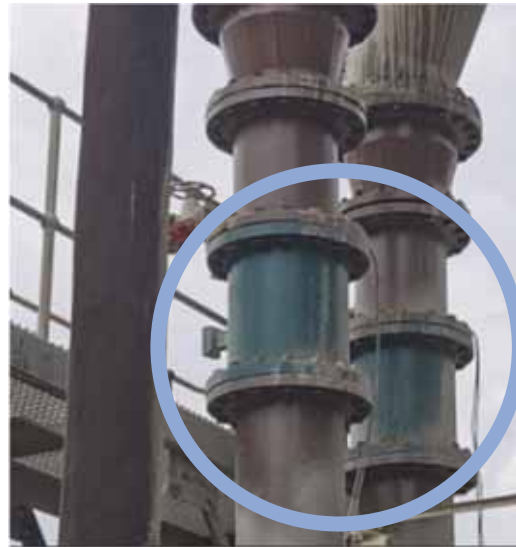
Slurry mag meters
